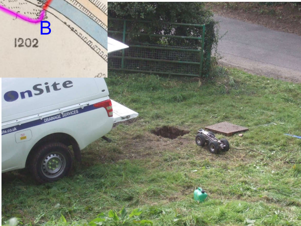
23. After the desilting, a photographic survey was done to check the culvert. This photo shows the Chamber's access manhole and the camera trolley.
