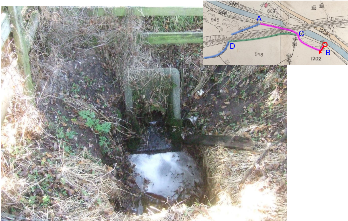
20. View into the access shaft showing the pipe outlet and inlet for the culvert.
