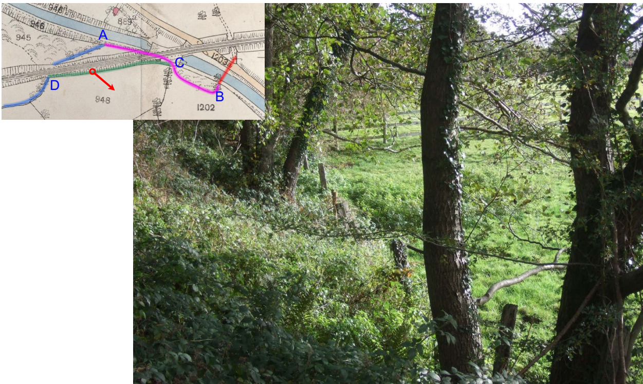
12. Near D, looking along the railway embankment. The Pipe Inlet, installed by British Railways, is somewhere in this vicinity, but the area is now so silted up that it cannot be seen. The Post and Rail Fence in the centre ground is a new boundary established in the field (no 948) and marks a change of land ownership.
