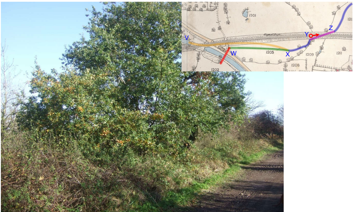
29 The outlet of the culvert (Z) is located some 40m distant further along the railway at the base of the embankment by the oak tree.
